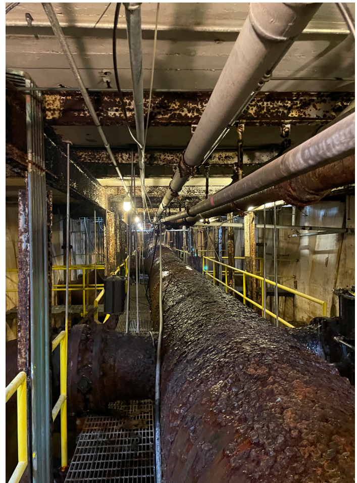
Pipe Gallery for the Sycamore Filter Basins at the Carrollton WTP
